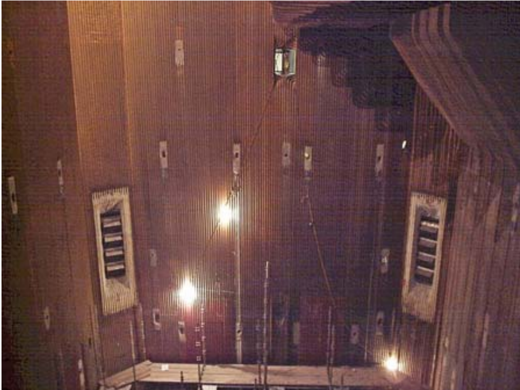
3. How low can you go? Rawhide Energy Station recently completed a low-NO x burner upgrade that included adding overfired air ports (shown on left and right of the photo). Also shown are the Zolo BOSS 2 1/2-inch-diameter laser ports added for in situ combustion properties measurement. Courtesy: Platte River Power Authority
