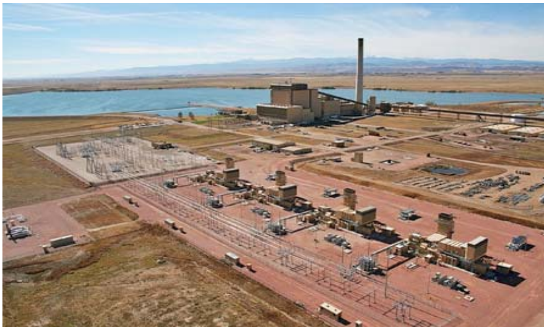
2. Mixed-use site. The Rawhide Energy Station includes four 65-MW GE Frame 7EA natural gas-fired turbines. A new 128-MW GE Frame 7FA turbine (not yet built when this photo was taken) was commissioned on July 23. Courtesy: Platte River Power Authority
